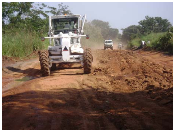
UNV heavy duty drivers and mechanics assisting the construction of the Yei – Kaya road
